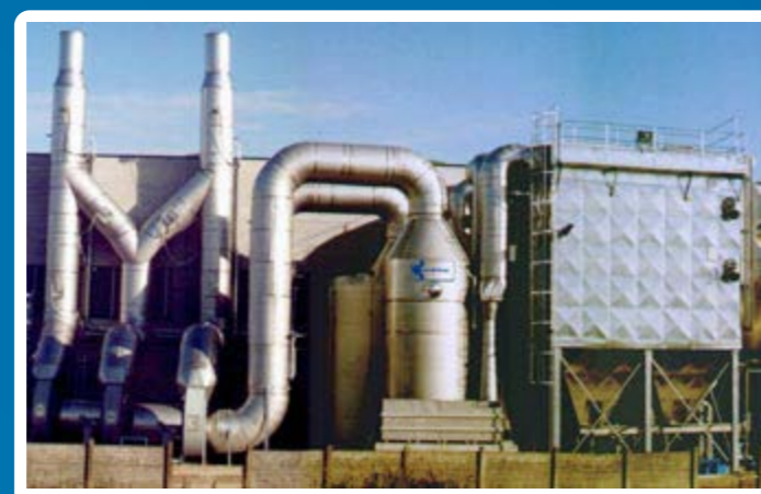
DUSTS AND AMINES TREATMENT FROM COLD-BOX DEPARTMENT ABBATTIMENTO POLVERI ED AMMINE DA REPARTO ANIMISTERIA COLD-BOX
